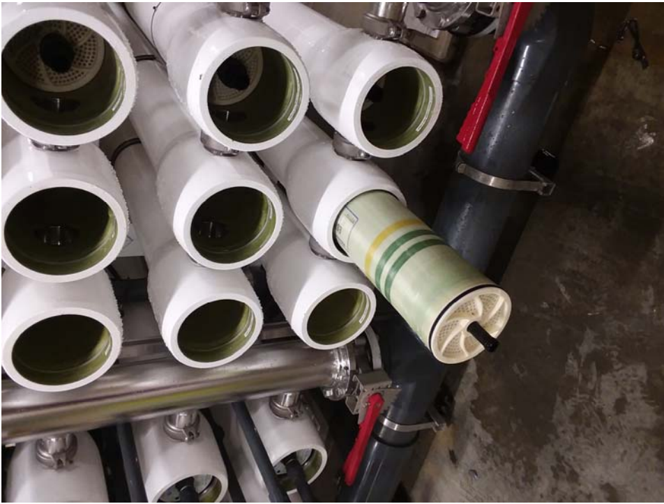
RO membrane element being installed in the pressure vessel located on the skid unit.
