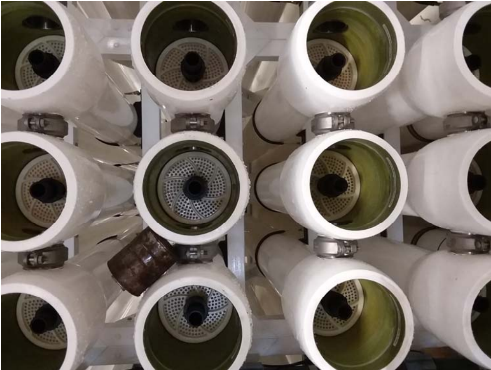
Open end cap of the pressure vessel with an installed RO element. Each skid unit is designed to treat 2.2 million gallons of water per day (MGD).
