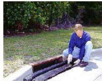
Drop inlet protection
