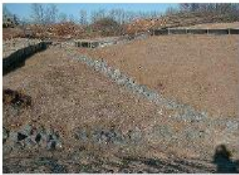
Riprap can be used to stabilize drainageways and outlets to prevent erosion
